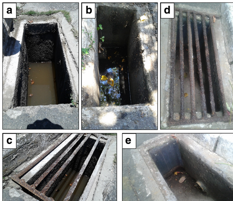
Fig. 2 Typical storm drains surveyed in Piatã neighborhood in the 2015 pre-intervention period (a, b, c) and in the 2016 post-intervention period (d, e), in Salvador, Brazil
